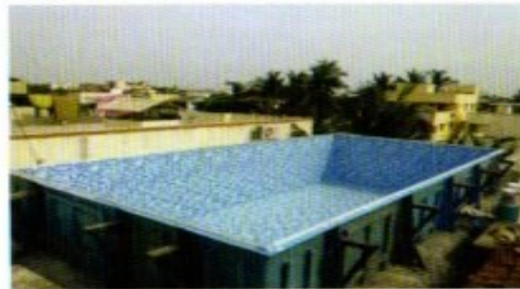
2. Second Step : For above ground pool the liner placement along with lights, filter and pool ladder.
