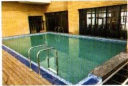
Overflow Prefab Swimming Pool at HOLIDAY INN
